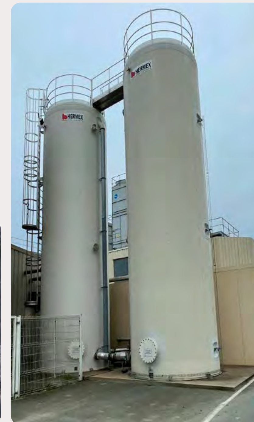
Two water tanks of 75m 3 at our site in Gourin, to store the site's hot water. The water is heated with residual heat
