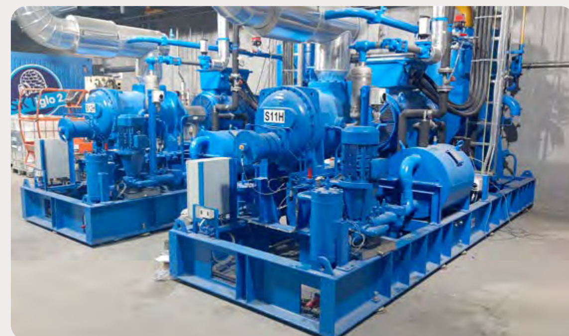
Capturing the residual heat from the cooling oil in our compressors to generate warm water for cleaning purposes
